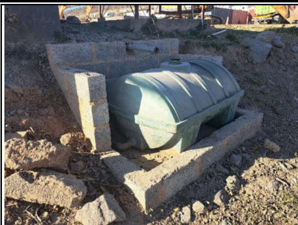
Size of bund to be increased and the bund to be sealed. Pipe to be lengthened
