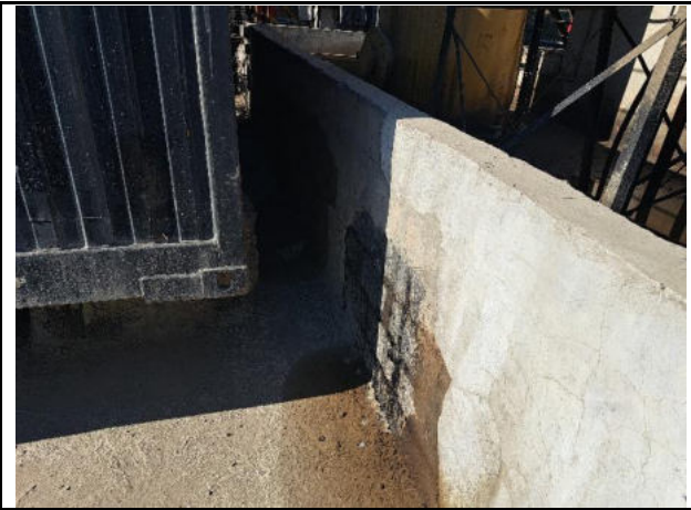
Bund to be sealed
