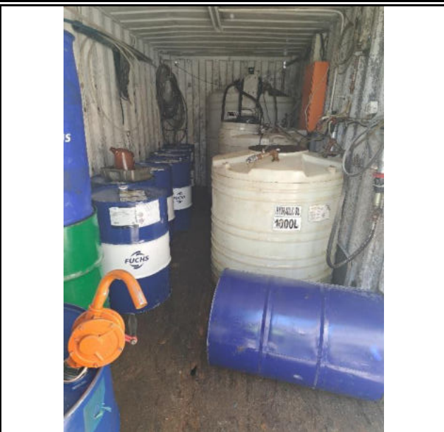
Floor of the oil store to be replaced by an impermeable lining
