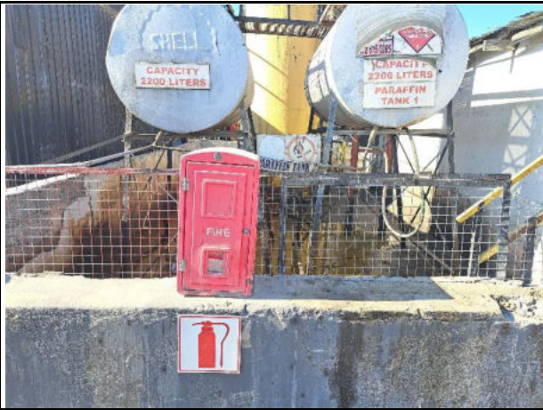
Fire extinguisher on site
